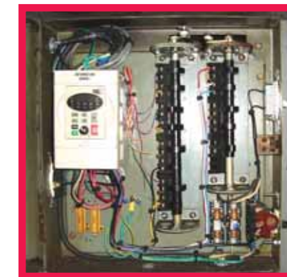
Figure 5, Completed Control Cabinet
